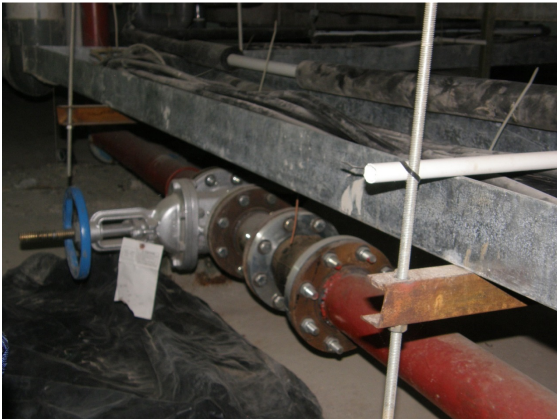
Photo 12 Flexible service joints in the Public Works Building. Photo: Phil Glassey, GNS.
