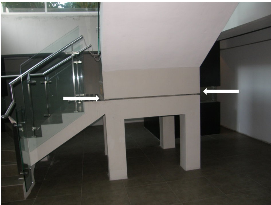
Photo 8 The stairs from the basement to the lobby are cut along the isolation plane (arrowed) to allow them to move with the isolation system. Photo: Phil Glassey, GNS.
