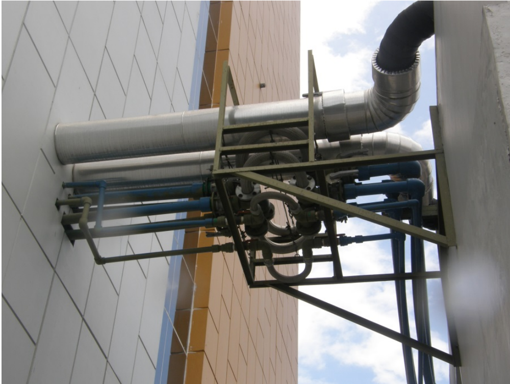
Photo 9 Services to the Hotel have flexible joints that allow for movement during earthquake shaking. Photo: Phil Glassey, GNS.
