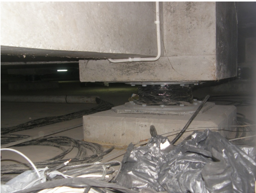
Photo 14 Base isolator beneath the Governor's office. Photo: Phil Glassey, GNS.
