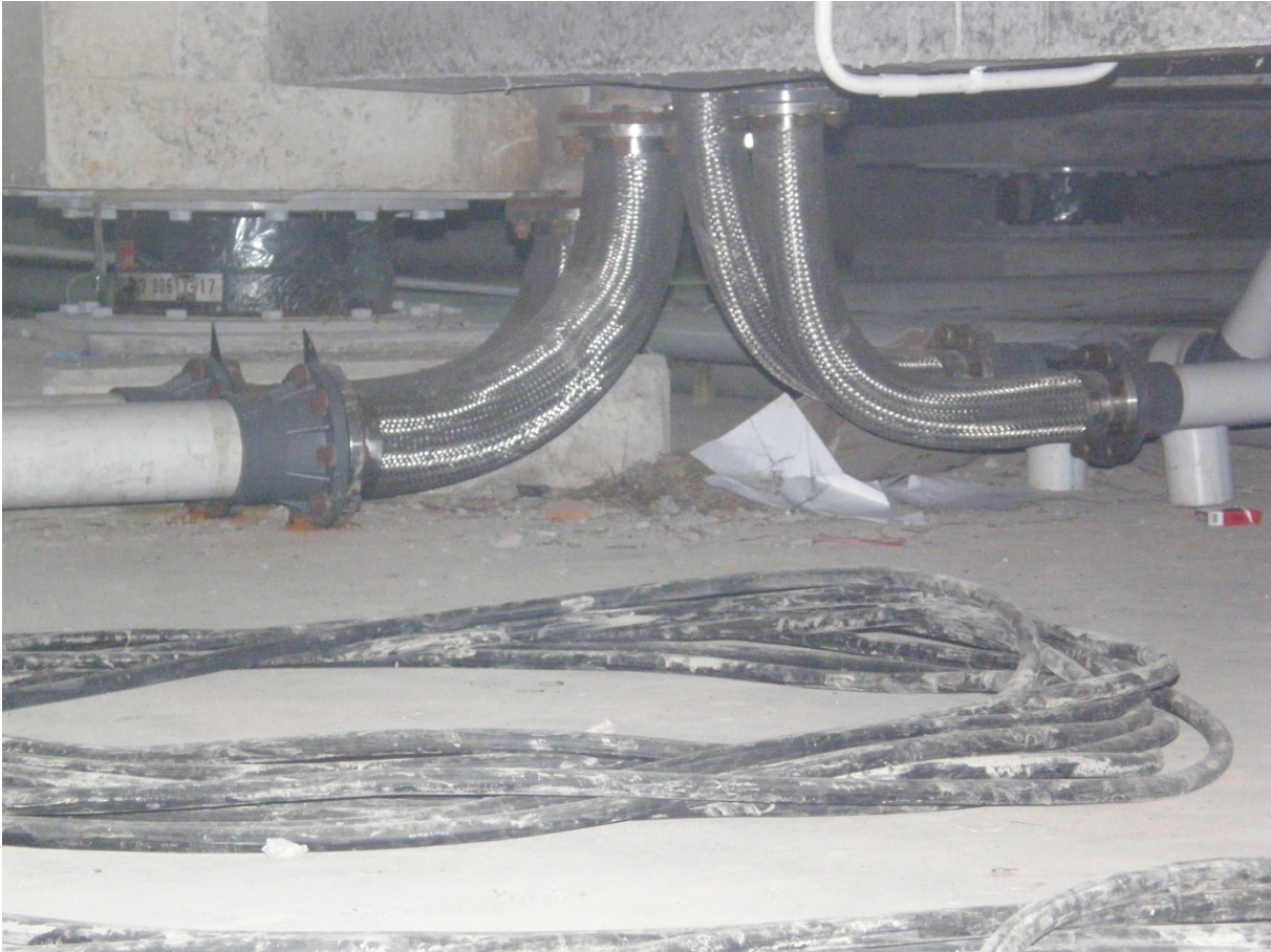
Photo 15 Flexible service joints into the Governor's building. Photo: Phil Glassey GNS.
