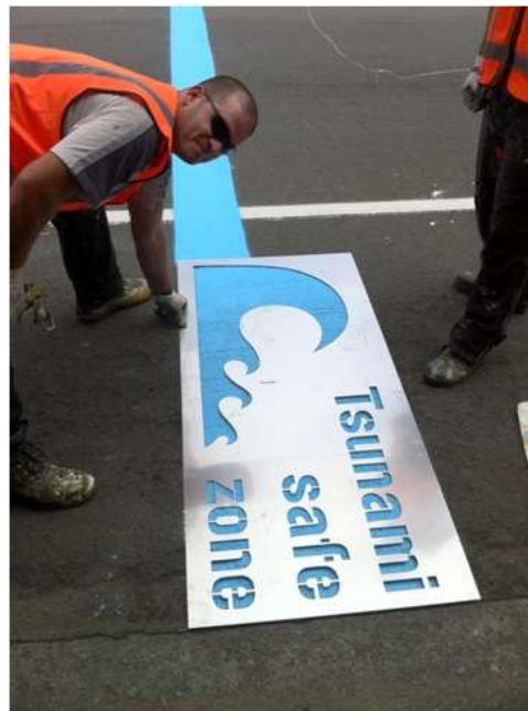
Figure 2: A contractor working on an instalment of a 'blue line' in Wellington, New Zealand.
