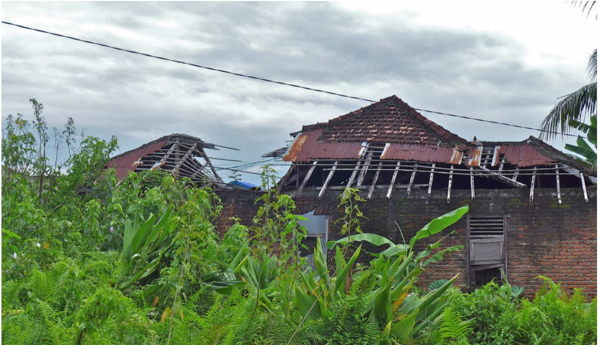
Building damaged in 2007 earthquake
