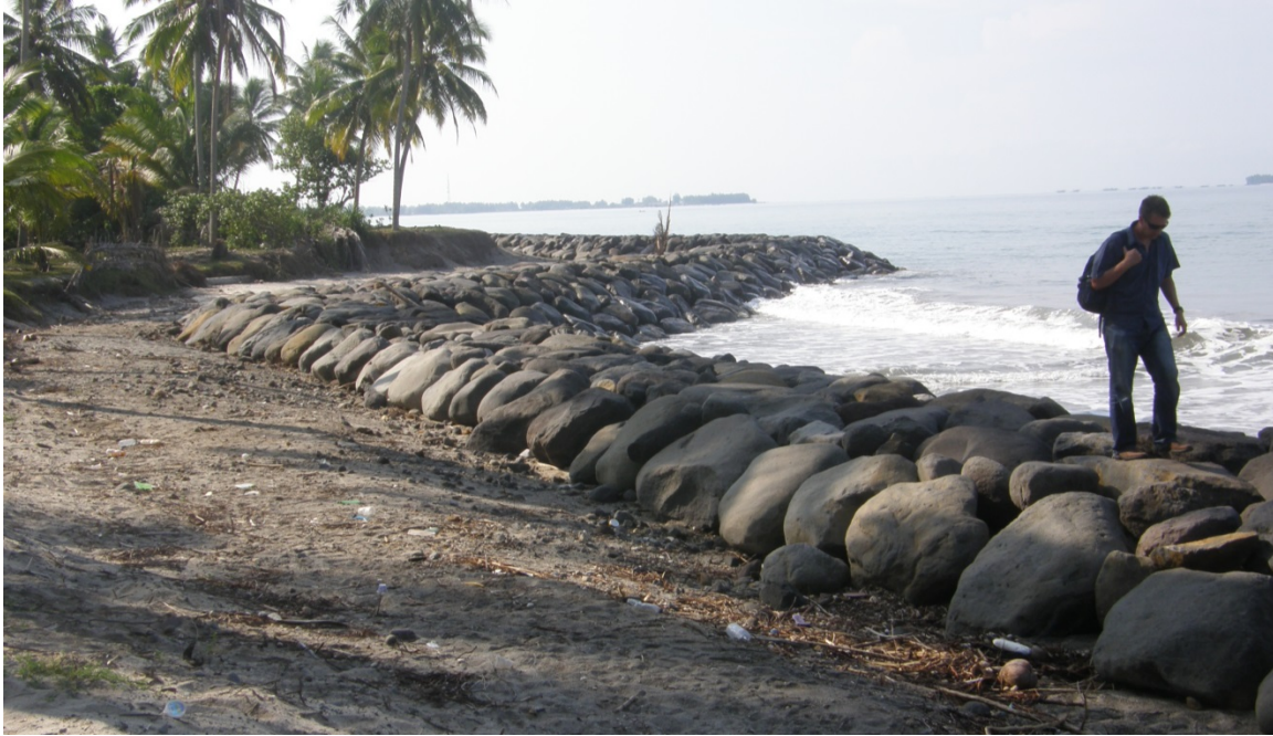
Erosion behind new erosion rockworks at North Tiku beach
